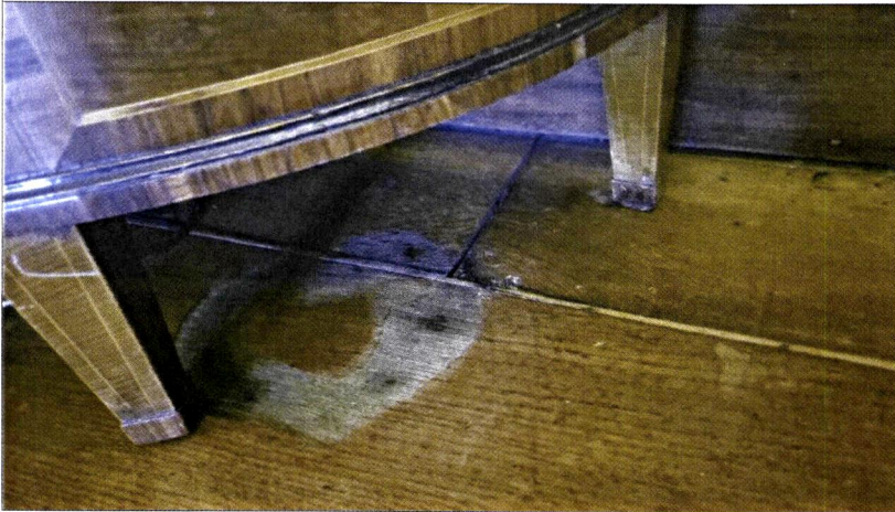
Music Room – historic water damage
