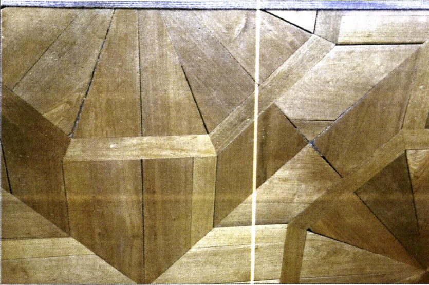
Saloon, shrinkage, losses, inappropriate and failed repairs
