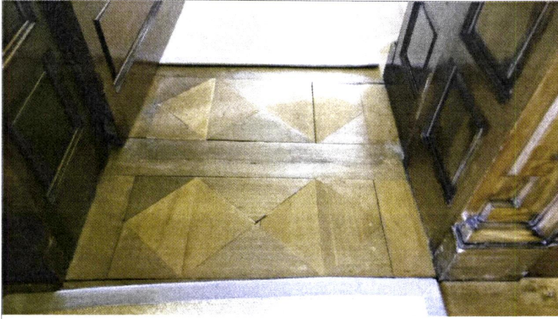
Music Room – threshold with shrinkage gaps and wear patterns
