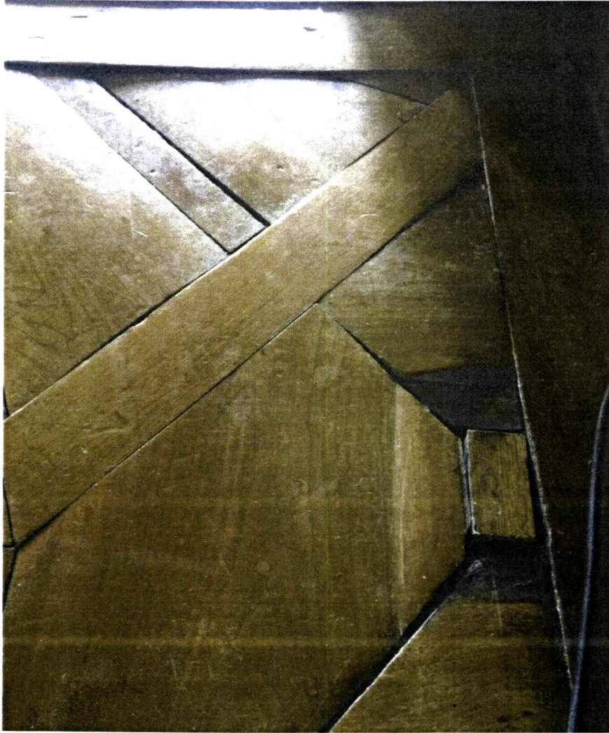
Misalignment of timbers indicating distortion of substructure
